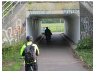
View of Long Road subway. A subway of this size may be a preferable alternative to widening the existing way under the railway bridge.
