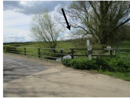
Option iv— Private Road leading to the private bridge (Marked with arrow) seen from Grantchester side .
