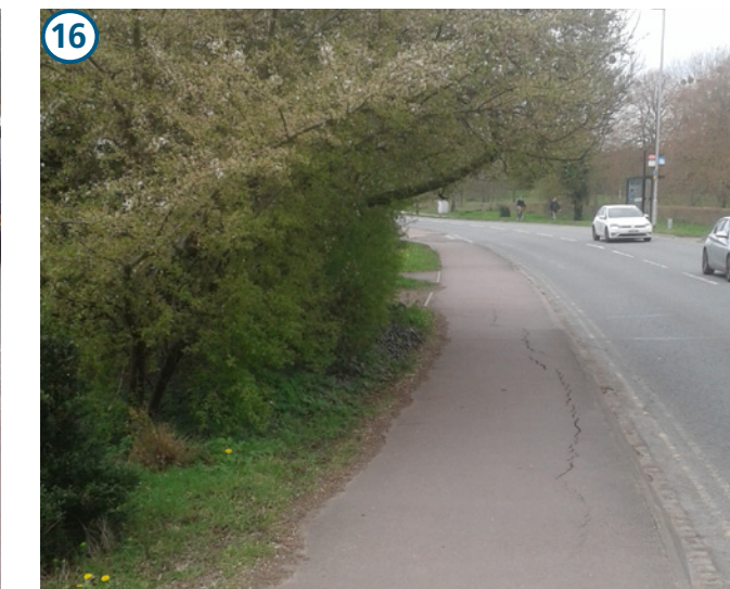
16 Wilberforce Road to Bulstrode Gardens - looking West Some trees on 3rd party land will need to be have canopies lifted to ensure sufficient space and height for cycle route
