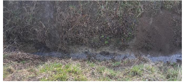
Figure 5.1.1-72 – Evidence of rats using banks
