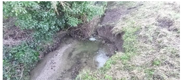
Figure TR5.1.A-6 – Bank Erosion
