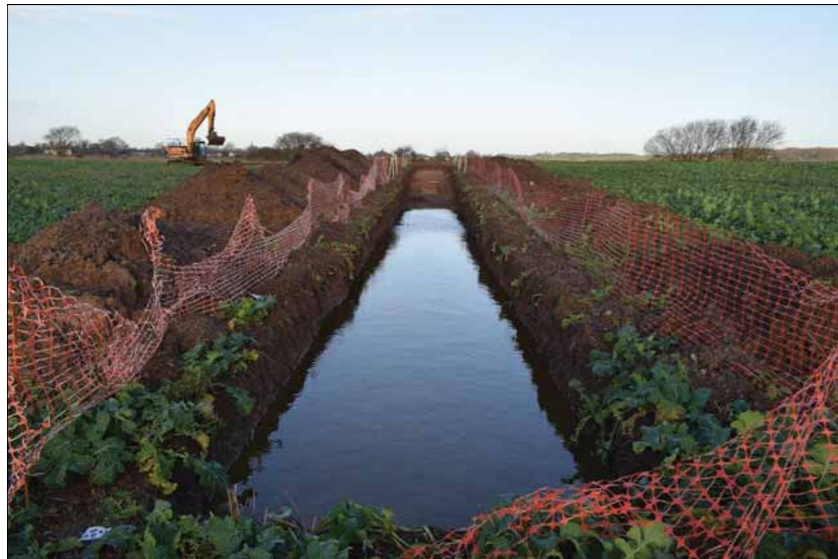
Plate 28: Trench 73 flooded, Field 7b, looking north-west
