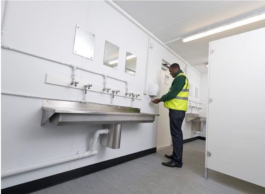
Figure 4: Typical washroom / toilet facilities
