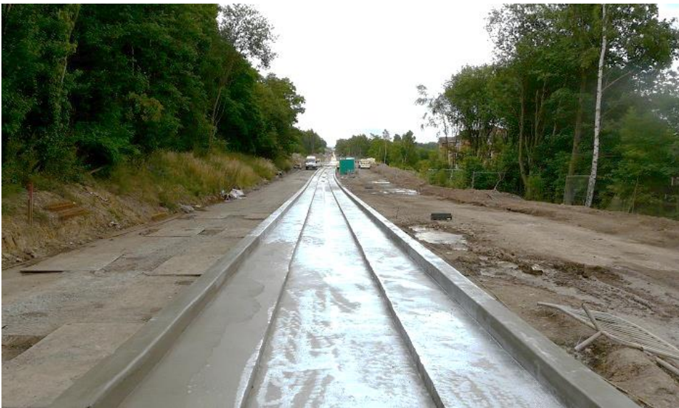
Figure 6.2: Slip formed kerb guided busways – Leigh-Salford-Manchester Bus Rapid Transit scheme during construction
