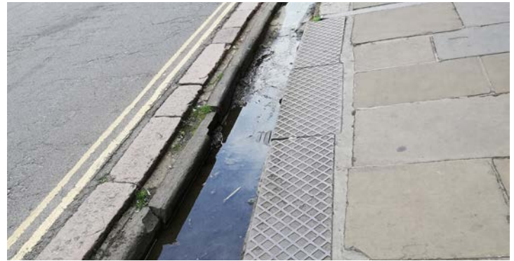
Image 24: Lack of Quality & Consistent Materials
